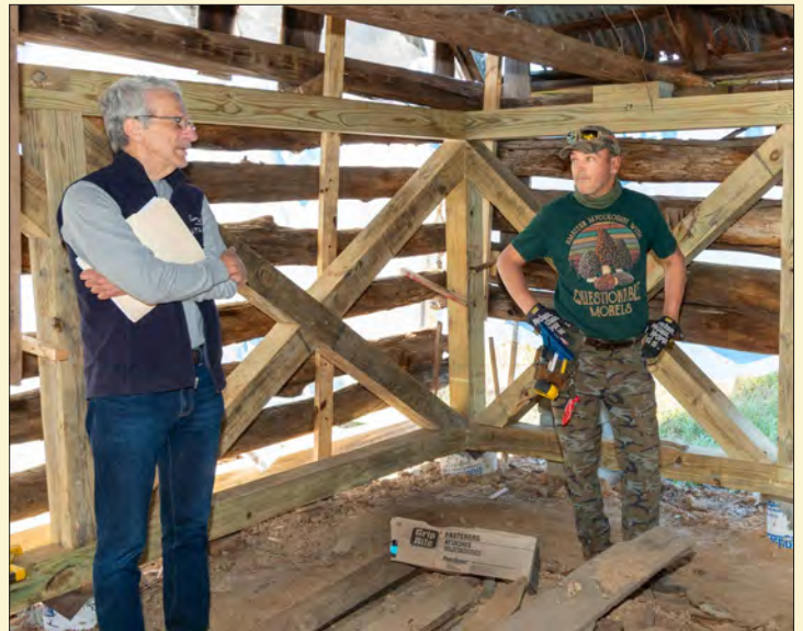
Greg Bowen at the Holly Hill barn stabilization project, with preservation contractor Jeff Thompson of Colonial Woodwrights Inc. Photo by Carl Fleischhauer
