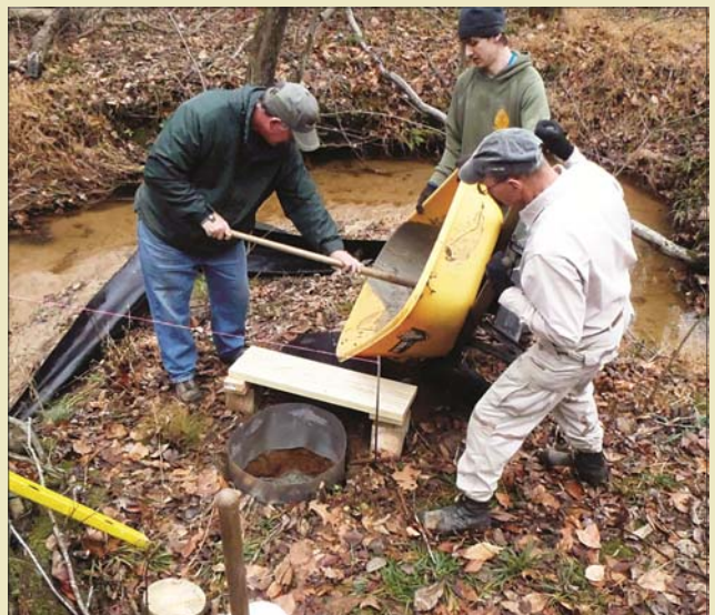
Left to right: Ron McClain, Ian McClain, and Ken Romney installing bridge pilings.
