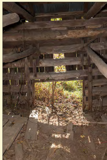
One of the small openings that provide access to the interior of the log barn.
