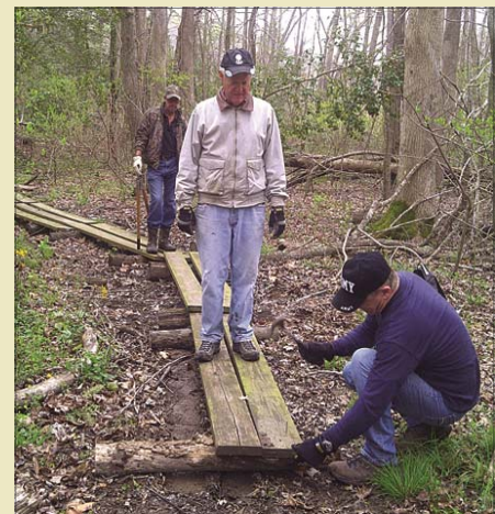
Mark Stachnik, Ed Haack, and Mike Walls (left to right) making repairs to Parkers Creek foot bridges.
