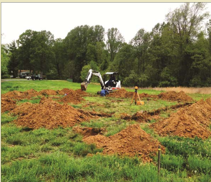
Foundation work provided by Gary Hammett and crew of Hammett's Building Services, LLC. Photo by Kady Everson.
