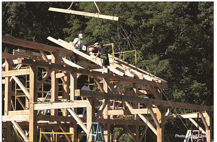
The construction crew installing rafters with the aid of a crane. Photo by Jeff Crespi.
