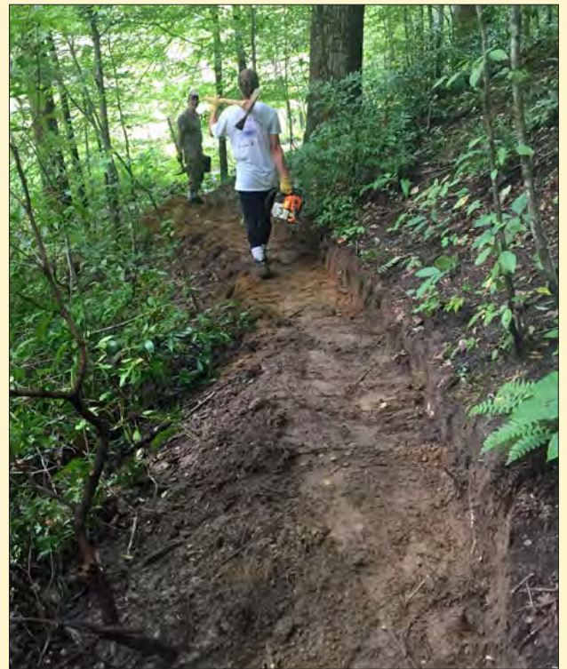
Side-legged re-route on the Ridge Loop trail. Trail is not yet backsloped.
